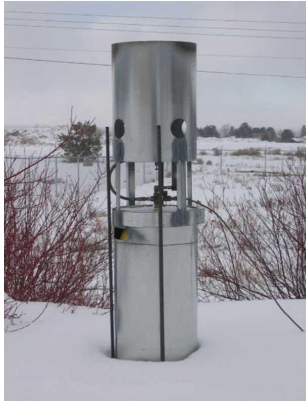
Fig. 5. Ground Based, Manually Operated Silver Iodide Generator
